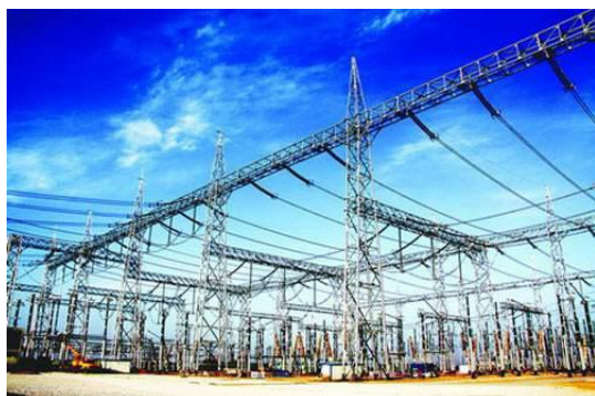
Intelligent substation control system
